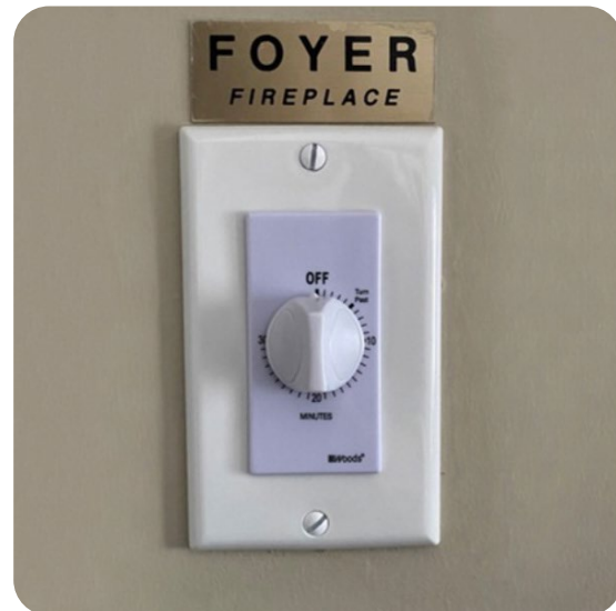
Control box to turn on the fireplace
