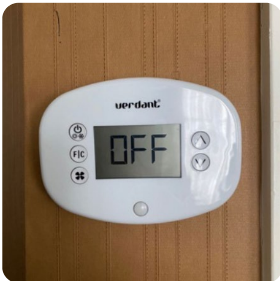
Air conditioning / heating control unit
