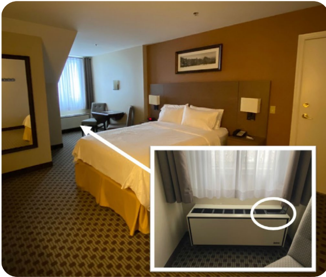
Hotel room (No fireplace) Control temperature directly on the machine
